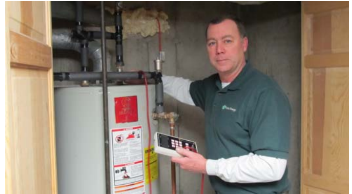
John Haithcock checking pressure and draft on water heater
